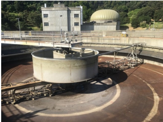
Secondary clarifier internal equipment
