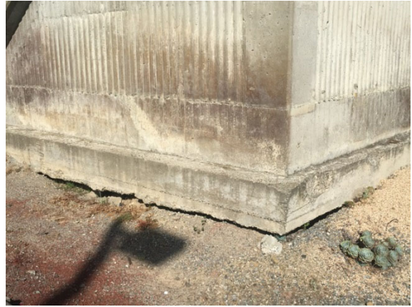
Exposed bottom of process tank
