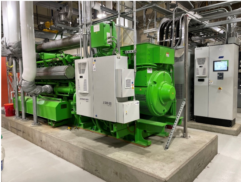
New cogeneration system
