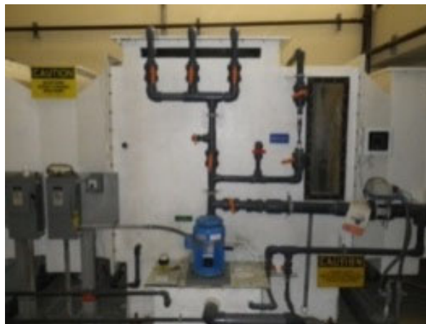
Solids Handling Building odor control scrubber
