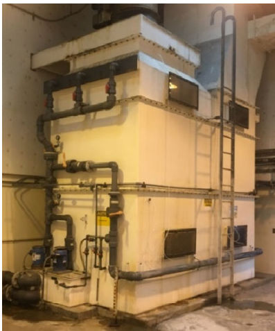
Headworks odor control scrubber
