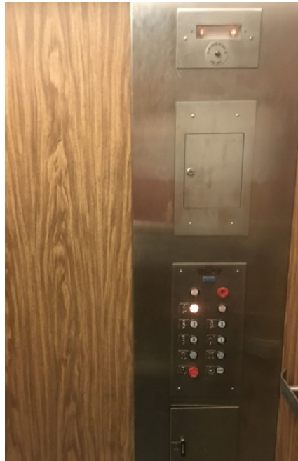
Elevator Control Panel
