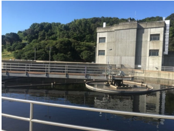
Secondary clarifier in operation
