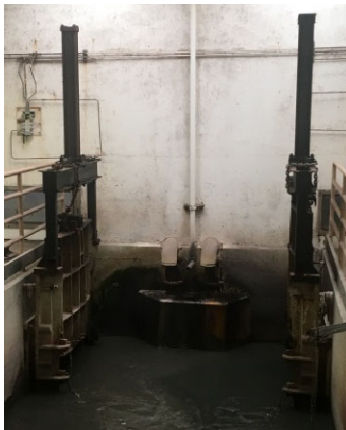
San Rafael and Ross Valley influent gates
