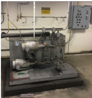
Hydraulic control system
